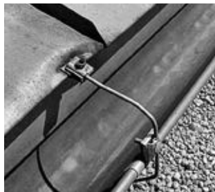
Fig. 10: Incorrect installation of lightning rod terminal to panel
