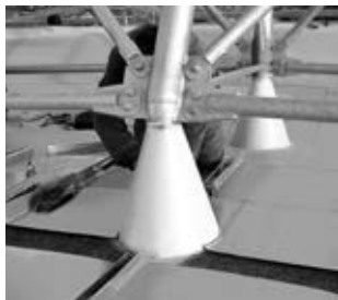
Fig. 6: Roof area with many penetrations
