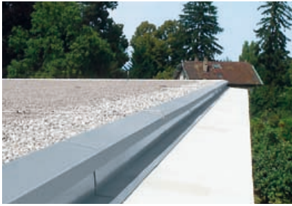
Connection to flat roof not visible from below
